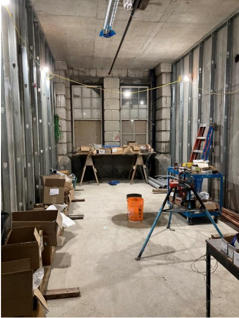
This is the back room of the new Archives, with former exterior pillars at back end remaining in place.
